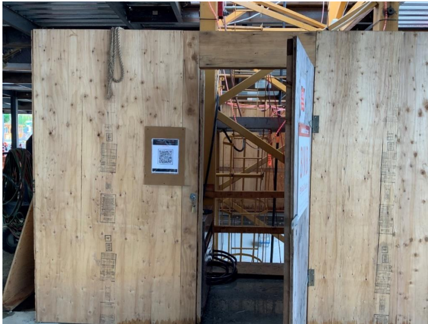
Figure 4 An access door is provided at the Tower Crane enclosure. These doors are equipped with a hasp and padlock that only the site management and Tower Crane operator are provided keys to. Doors should be locked up at the end of each day by site foreman during final walkthrough at the end of each day.
